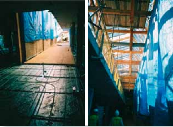
Left: Under-floor water pipe heating and rammed wall
