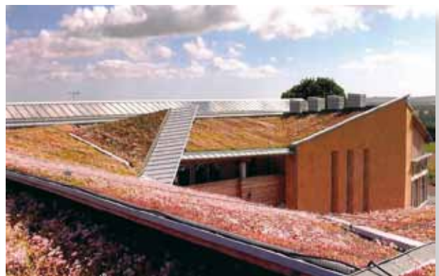
Sedum blanket green roof
